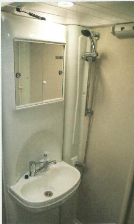
The basin and cabinet swing through 90 degrees to create a shower cubicle
