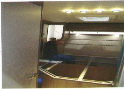
16 Meanwhile, inside the van, technicians are beavering away fitting bed mechanisms and doors, etc. The LED roof and reading lights are also fitted and working, as is the rising bed frame.
