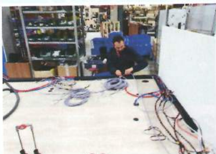
4 Rolling on its wheels, the embryonic tourer is towed along the production line by a pulley system. It stops at each workstation for a job to be completed. Here they fit vinyl flooring, pipework and cabling.
