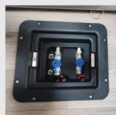
Access to the 'van habitation controls is via the floor
